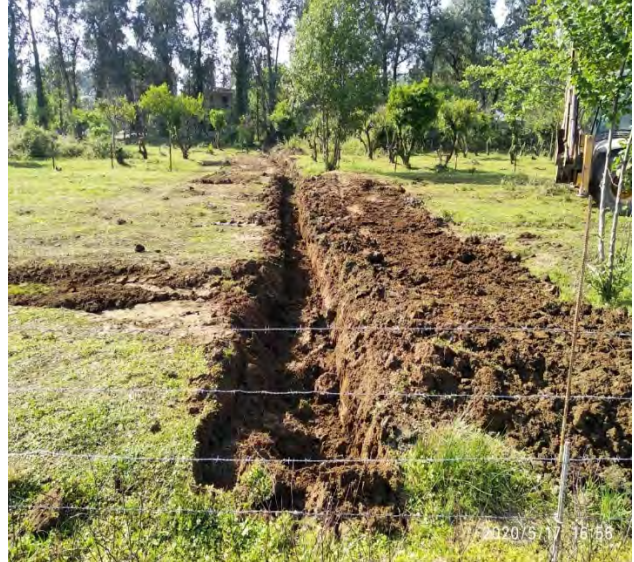
View of the land plot after the Contractor implemented channel cleaning activities
